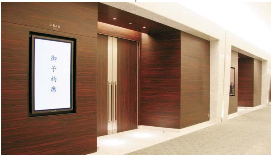
The plasma display installed at the entrance of each banquet room provides information. The displayed information can be easily changed by switching the content data. Previously, a signboard had to be produced for each event.
